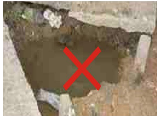
Unsuitable water accumulation
