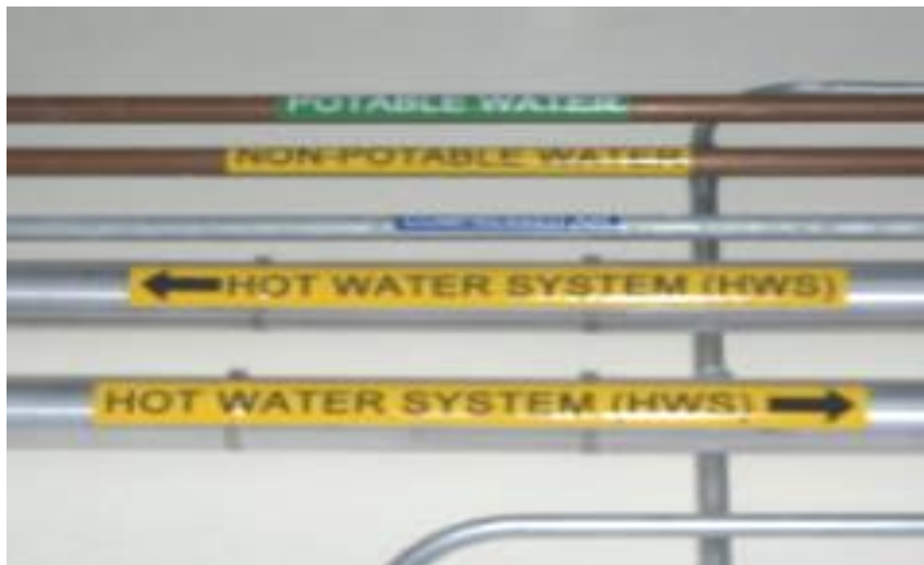
Separate pipelines for potable and non-potable water
