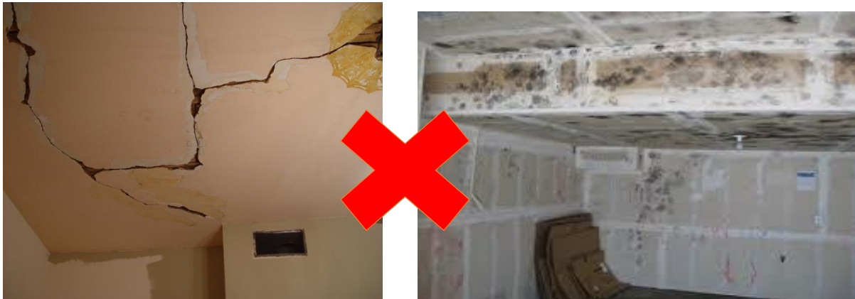
Wall and ceilings with crevices and mold growth
