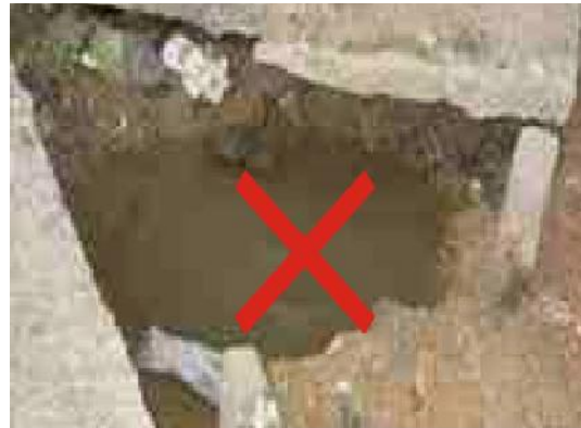
Unsuitable water accumulation
